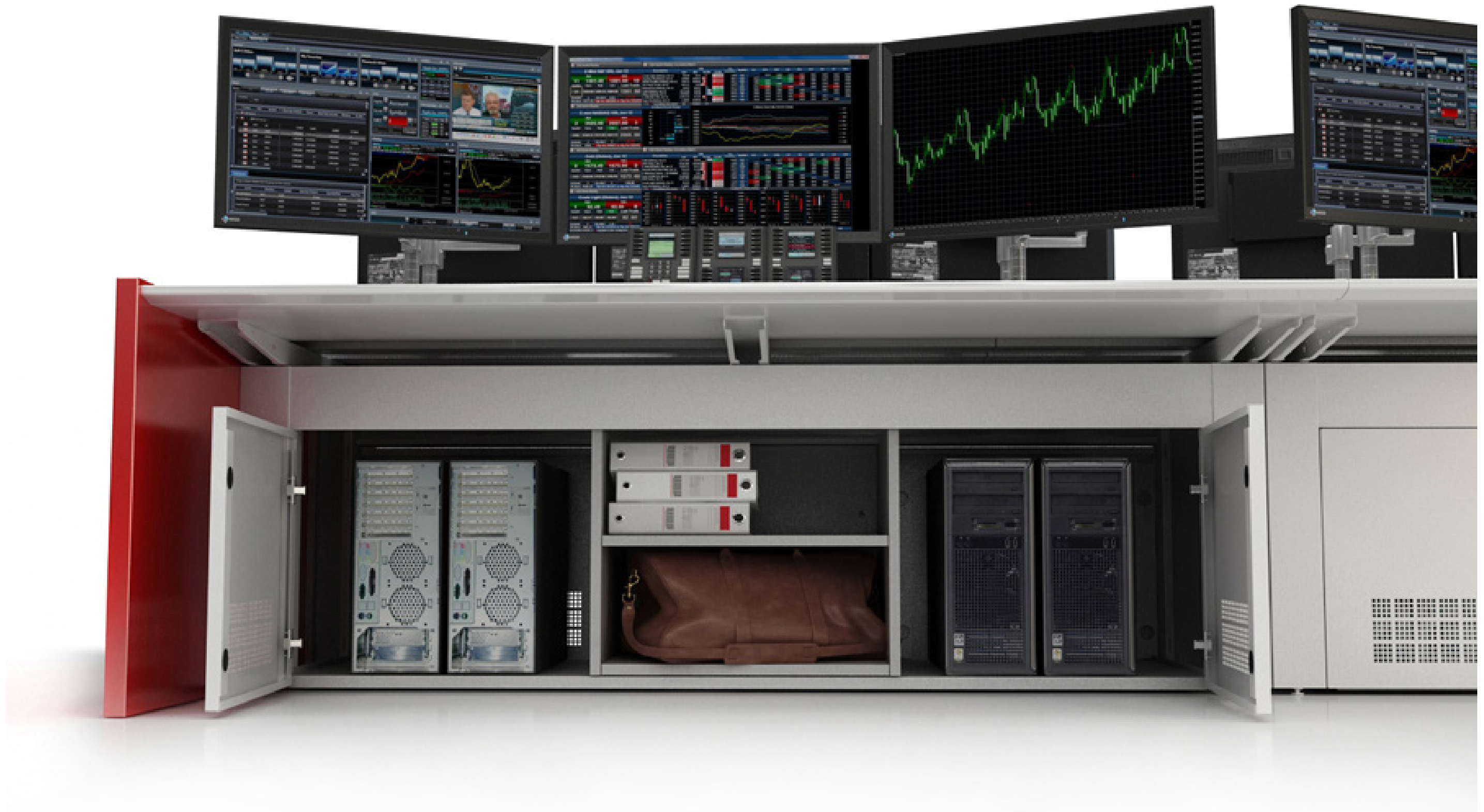
Hinged access door to CPU enclosure and personal storage space.
